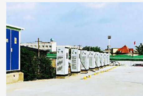
Super charging station
