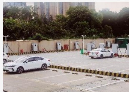
Super charging station
