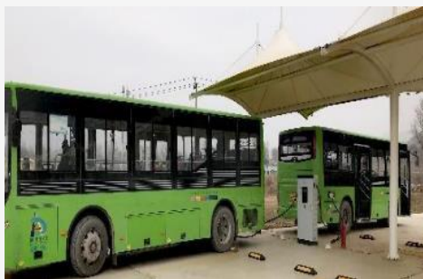
Bus Charging Station
